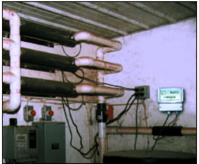
Triangular Wave Technologies Deposit Control System Installed Before Ultra Violet Disinfection System
